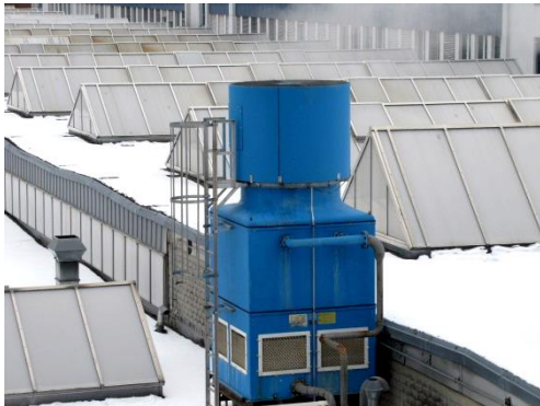
Example of a cooling tower used in industry
